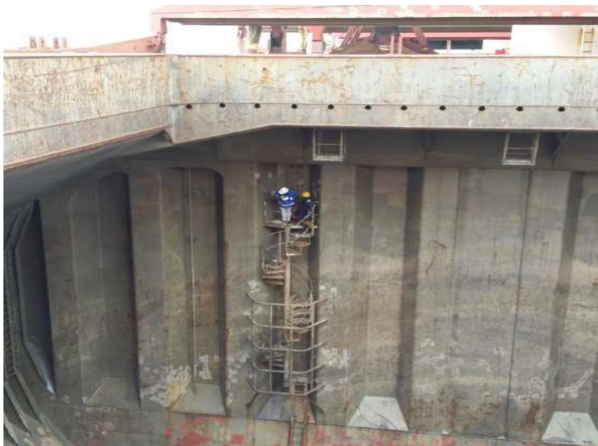
Figure 3.1/2: Australian Ladder and vertical ladder's landing platform at cargo hold no 3 aft entrance.
